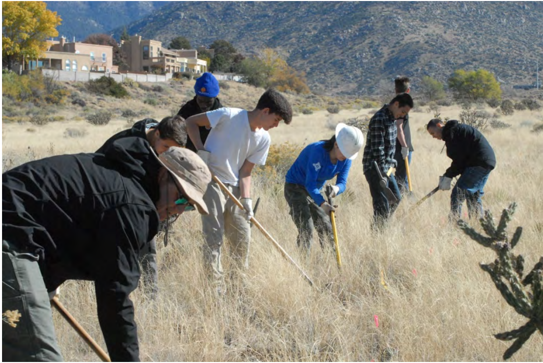
Trail construction project at BCOS by a student volunteer group led by OSD staff
