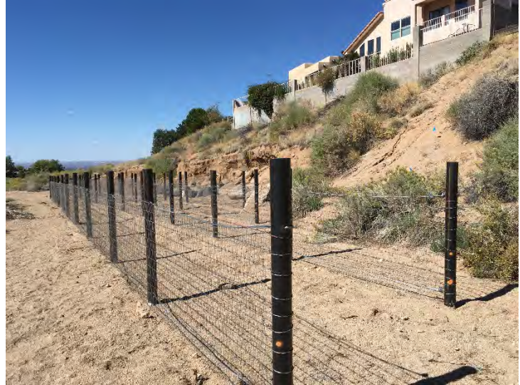
Erosion control system constructed by COA Hydrology in Bear Canyon West (Project 9)
