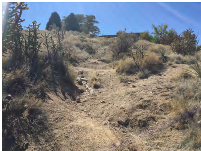
Photograph 2. Erosion from unofficial trails.
